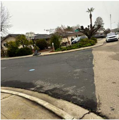
Missing stop sign, crosswalk and curb ramps at the Lynn Street approach to Irene Way.
